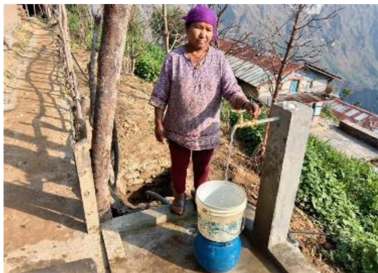
Figure 33 Beneficiary using newly constructed tap at Bokchen
